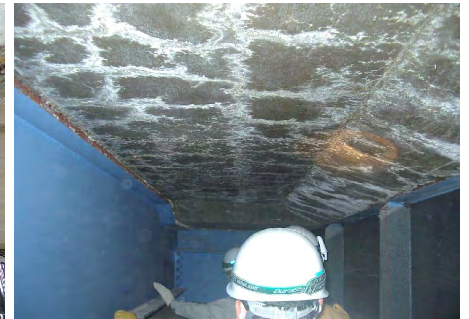
Concrete free lime
