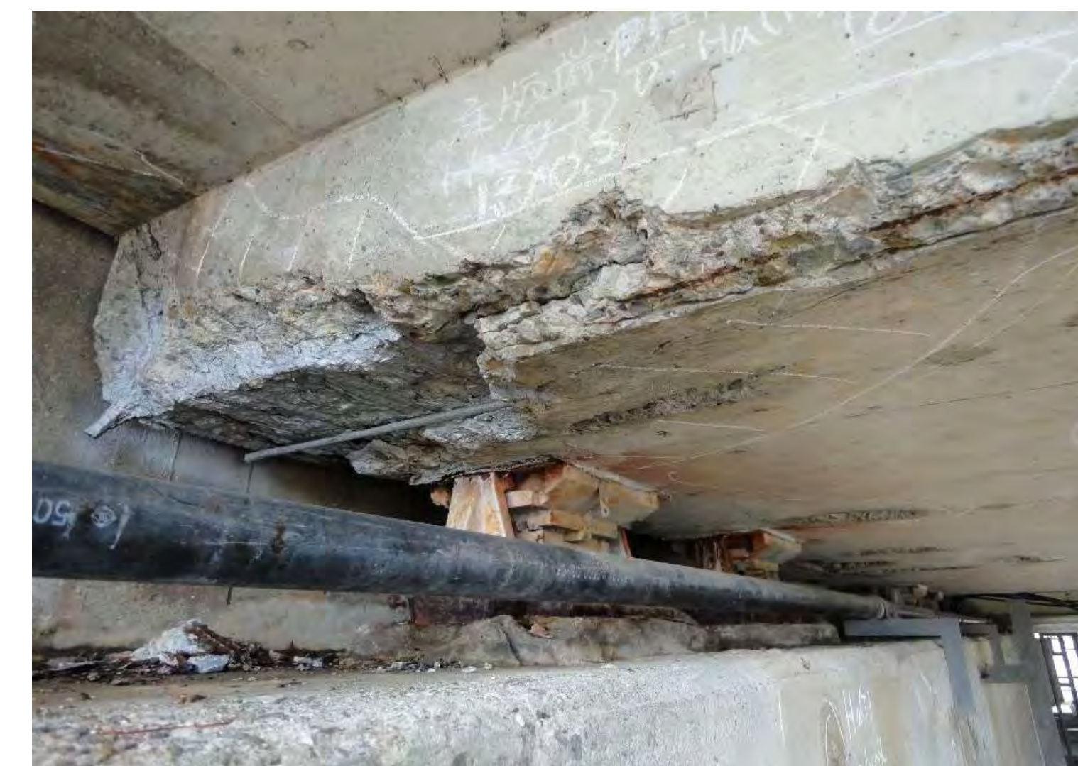
Concrete cracks and float
