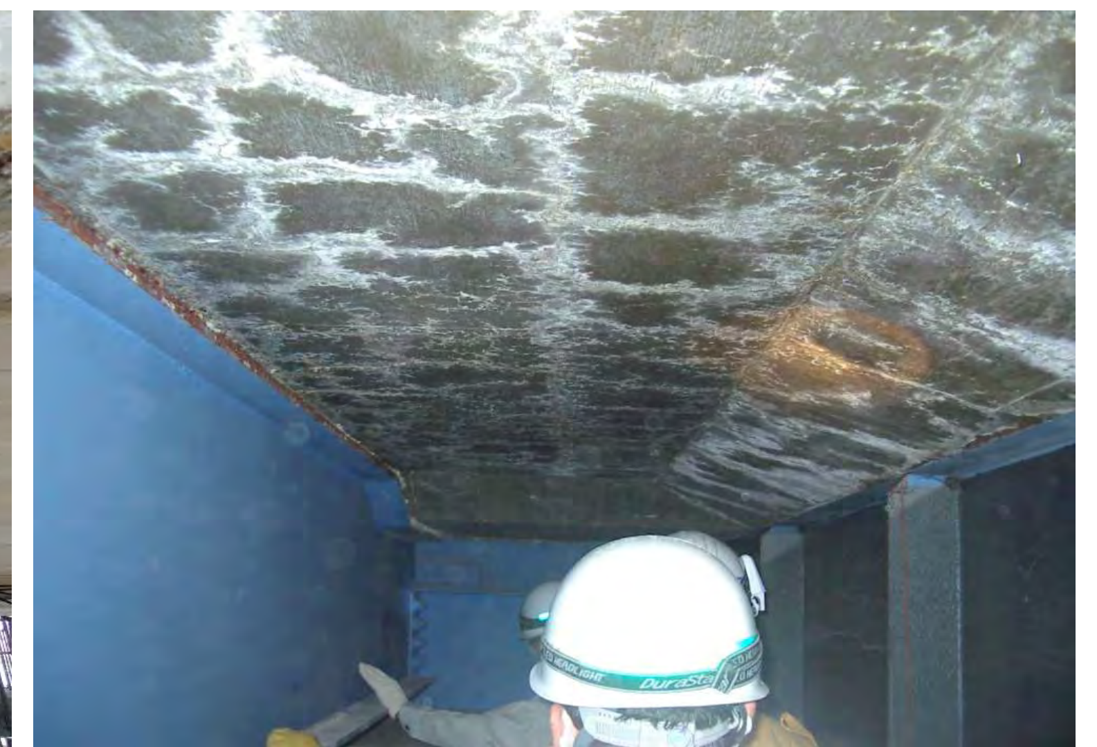
Concrete free lime
